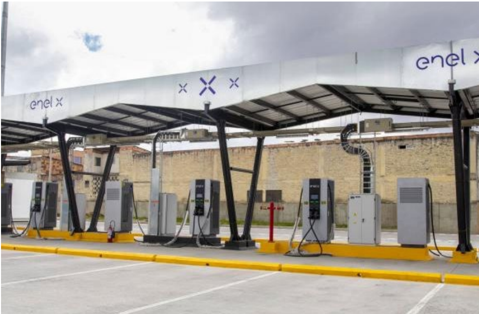
Figure 4-10 - Adequate garage with charging infrastructure in Bogotá'
